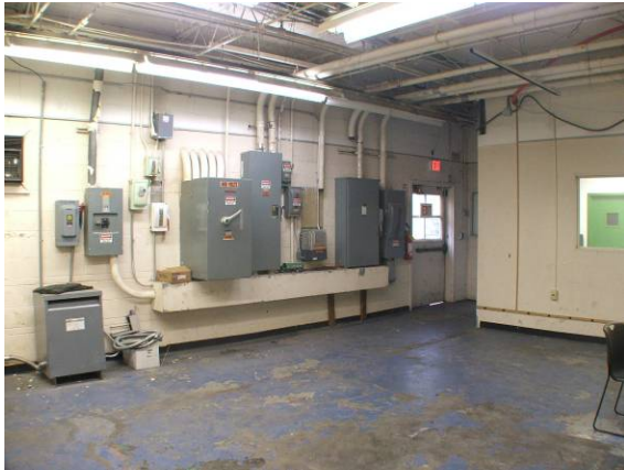
View of Electrical Room
